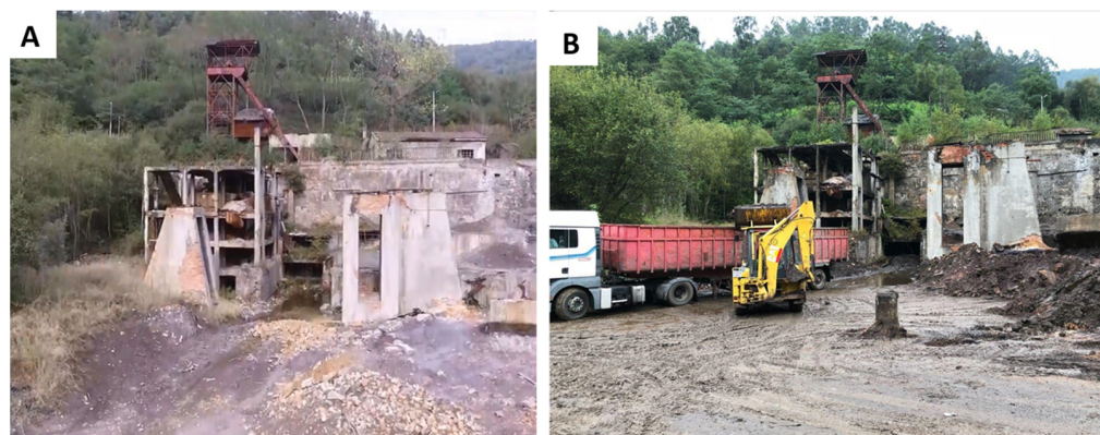
Figure 4. Demolition debris at El Terronal site before (A) and during removing works (B).
