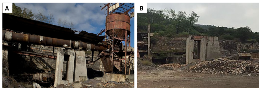
Figure 2. Metallurgical area in El Terronal before (A) and after (B) dismantling the roaster.
