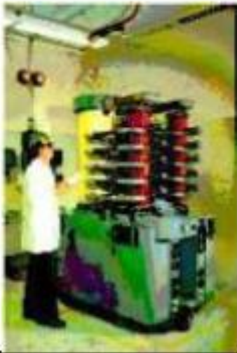
Mercury Arc Valve HVDC (Phased out)
