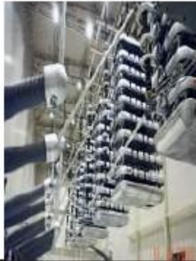
Thyristor Valve HVDC Classic
