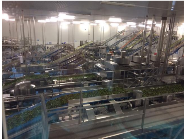
Figure 1. Distribution lines in a processing company (part of the production pipeline).
